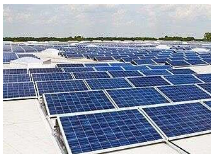
Fig.no.4 Solar Panels
